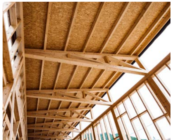
Figure 15 • Light Framing Roof and Wall Panels Used in Conjunction with Timber Trusses.
